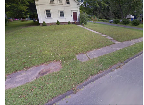
A sidewalk with significant uneven surfaces on Federal Street, rendering the segment non-compliant with ADA standards. Image: Google.
