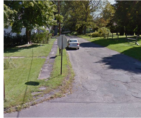
A narrow sidewalk segment on Hinckley Street that does not meet ADA requirements. Image: Google.
