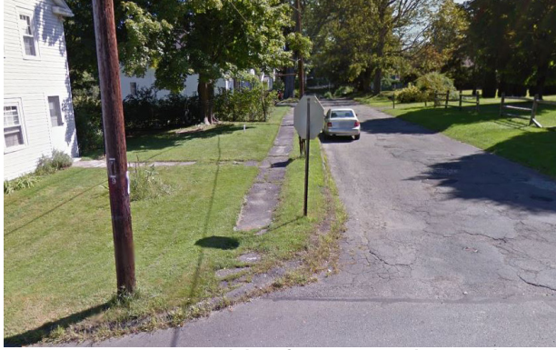
Figure 2.5: A missing (and therefore non-compliant) pedestrian curb ramp on Hinckley Street. Image: Google.
