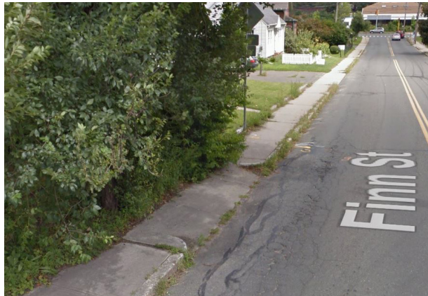
Figure 2.13: An example of a non-compliant (and defunct) curb cut on Finn Street just east of State Street. Image: Google.
