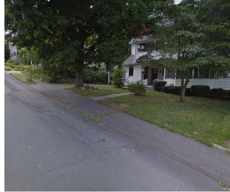
A segment of sidewalk that exceeds the ADA-accessible 2% maximum cross slope. Image: Google.
