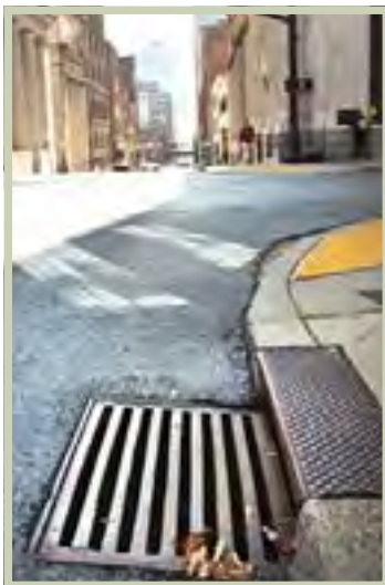
A bicycle-unfriendly sewer grate design in Nashville, TN. These should be avoided at all costs.;
